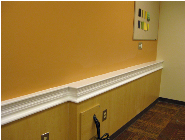
FIGURES 16-19 (clockwise from top left). Val (upper left in red shirt) and her team during the demolition and build-back phase of the work. Patching and prepping of walls and installation of a new chair rail cap.
